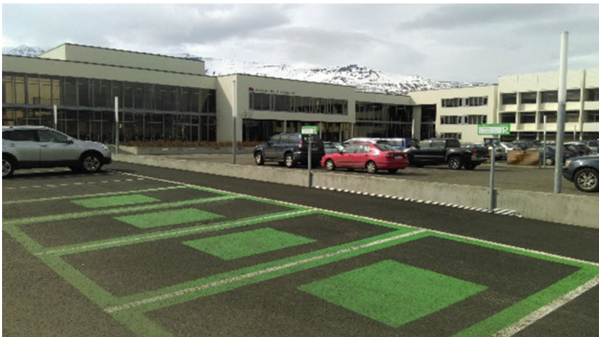
Fig. 21.1 Recharging spots at Akureyri University
