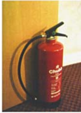
Fig. 5.8.6b: A fire door which has been propped open
