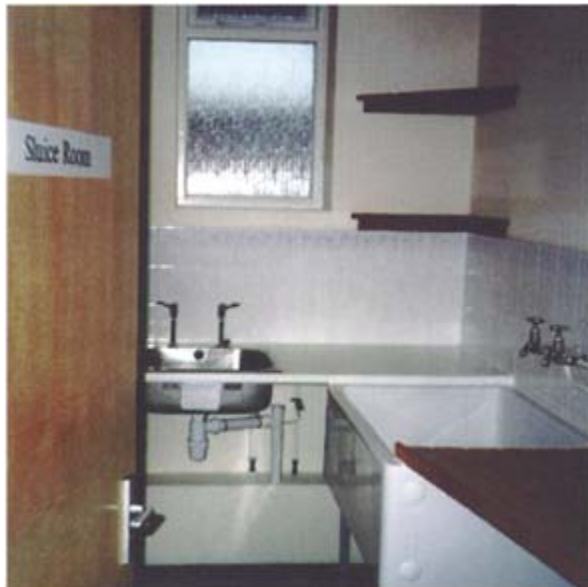
Fig. 4.5.2e: A sluice worn
