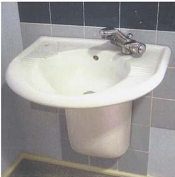
Fig. 6.2.5a: Wheelchair-accessible wash basin
