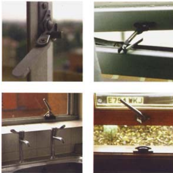
Fig. 4.3.2b: Inappropriate window details
